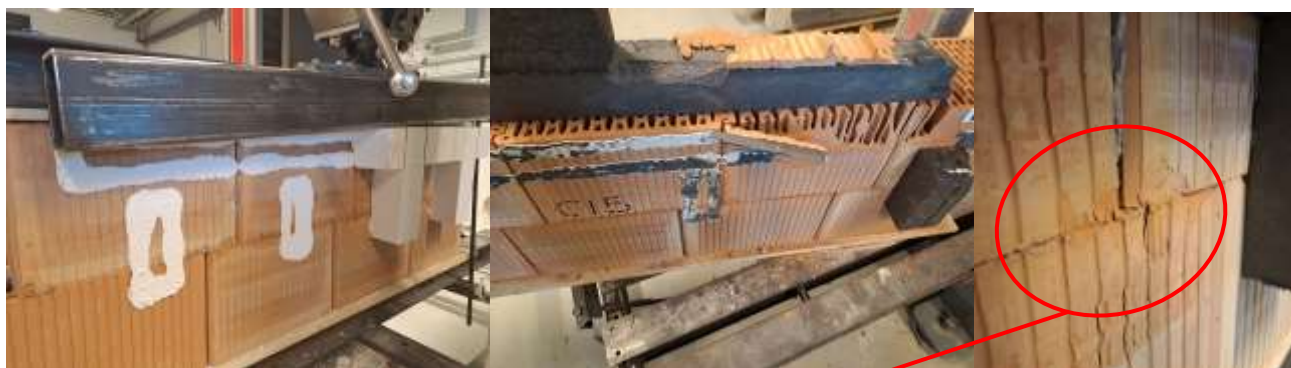
Fig. 11. KERATERM wall construction after tests. Cracks from tolerance flaws
